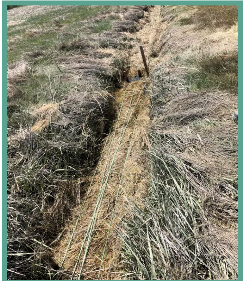
Ditch filled with salt-marsh grass, held in place with twine and wood stakes to collect sediment over time (Source: Wendall Waters / Wicked Local)
