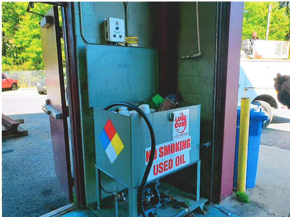
Waste Oil 'Remote Fill'
