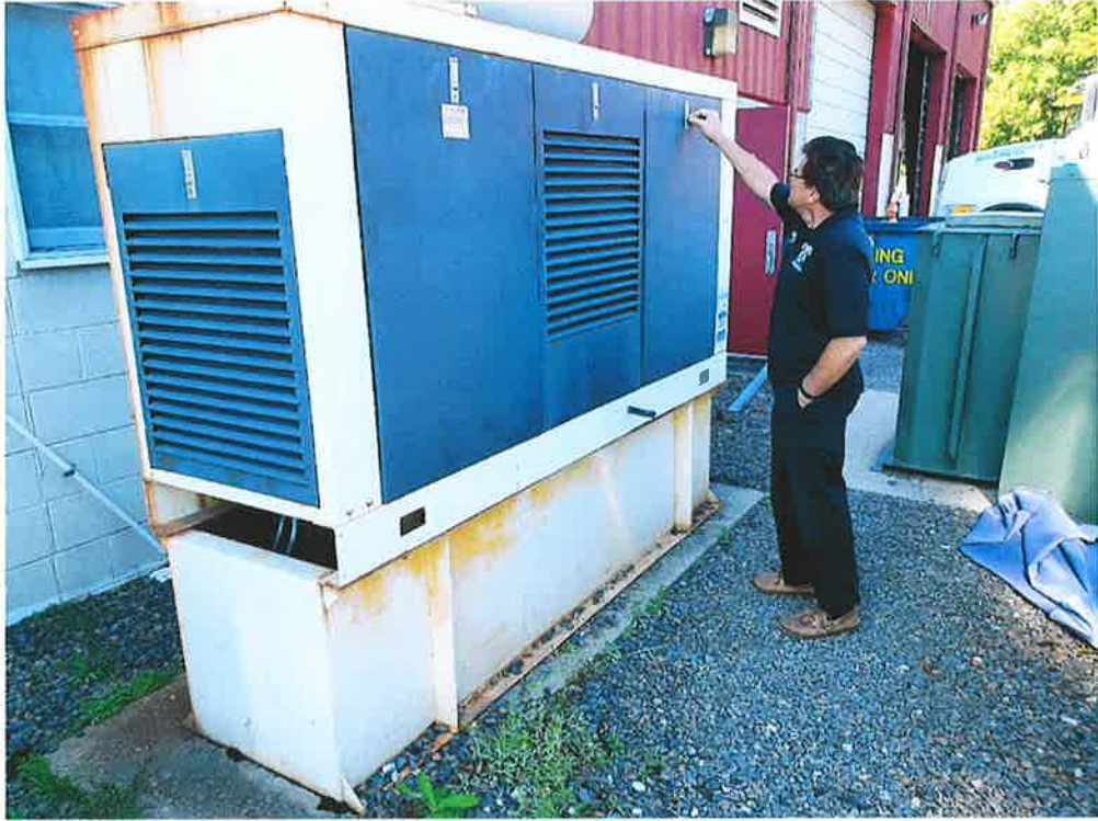
AST 4: 300-gal Diesel Fuel 'Belly Tank'
