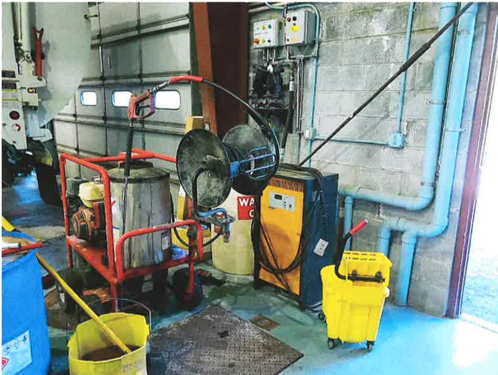
Oil/ Water Separator within Garage
